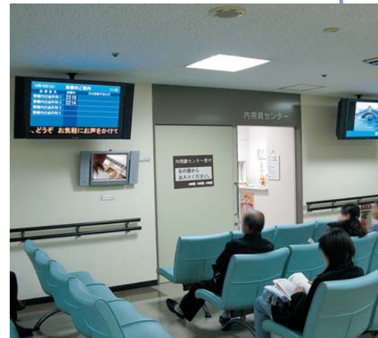
The display panel shows call numbers clearly. Since the panel displays the waiting list, it minimizes patient stress and allows everyone to check whether they have been called or not when, for example, they return from the lavatory. (The screen images in the photo are simulated.)
