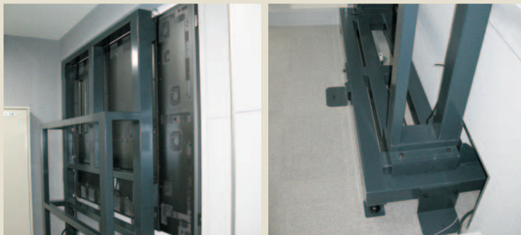
The display is mounted on a specially built frame in the machine room next to the AV hall (left photo). The frame has casters to allow movement, but they are normally fixed with stoppers (right photo). The machine room has air conditioning for the rear projection system, so it required no additional heat control measures.
