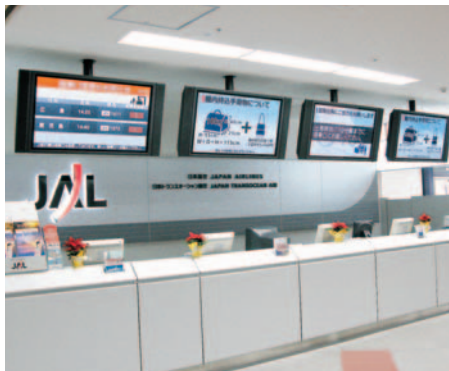
Multiple displays are installed at the counter for the added convenience of standby passengers.
